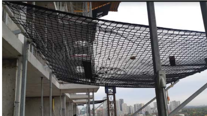
Figure 3: Safety Net at Dundas Square Gardens to Catch Fallen Materials and Debris [8]
